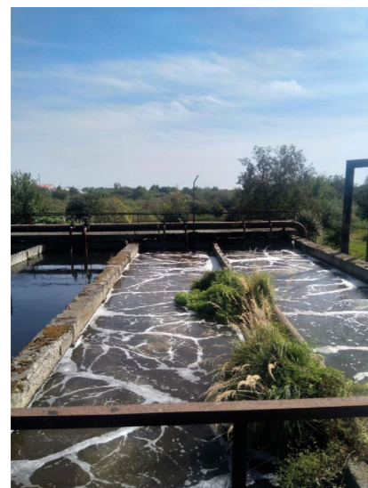
Waste water treatment plant, Lvivska Oblast, September 2024
